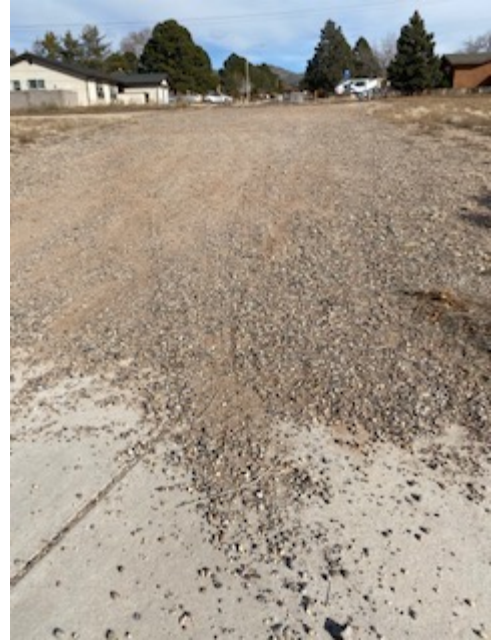
Rio Arriba Exit ramp condition
