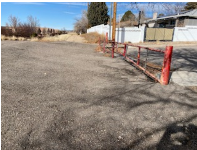
Raton Emergency Exit Gate from Juan Tabo Hills side. Part of the berm shown on the left.
